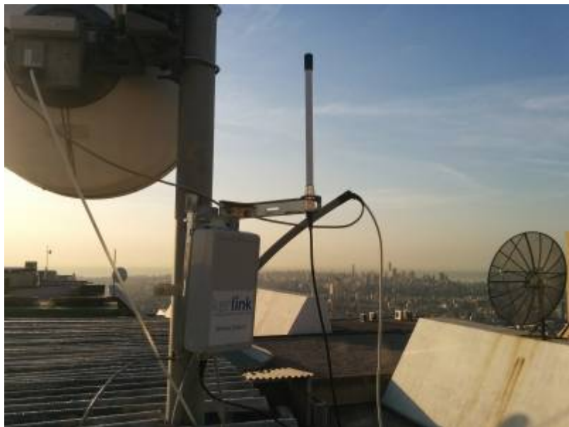
Figure 2. Outdoor antenna at ESIB-USJ
