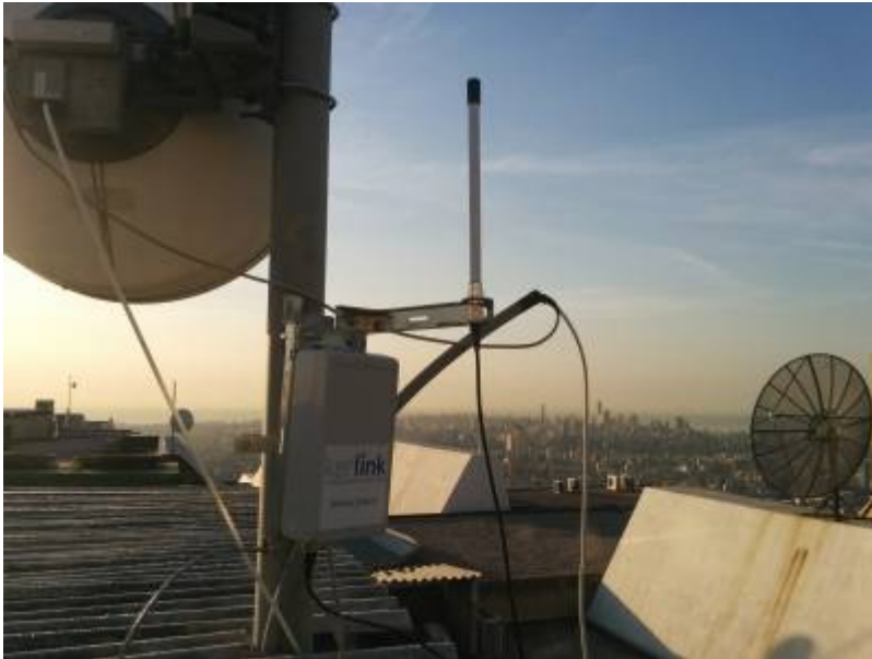
Figure 2. Outdoor antenna at ESIB-USJ
