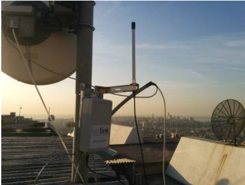
Figure 2. Outdoor antenna at ESIB-USJ
