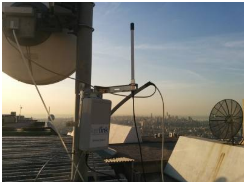
Figure 2. Outdoor antenna at ESIB-USJ
